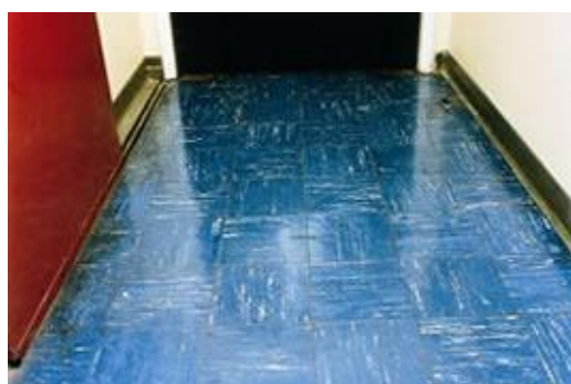
Asbestos containing floor tiles in a corridor
