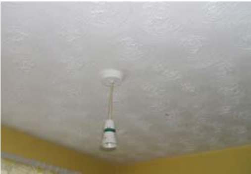
Asbestos textured coating
